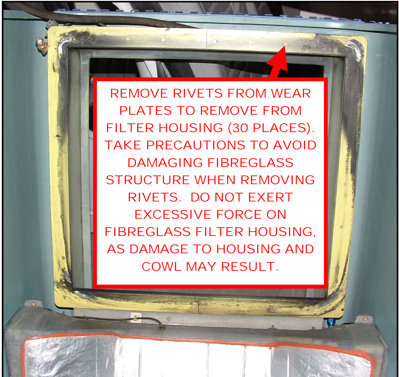
FIGURE 2 : VIEW OF INLET PLENUM WEAR PLATES FROM UNDERSIDE
